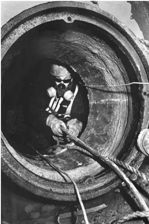
Figure 2-1. Many jobs require work in confined spaces, which requires specialized training and procedures, which are specified in the OSHA standard on Permit-required Confined Spaces (1910.146) (Photograph by Earl Dotter.)
